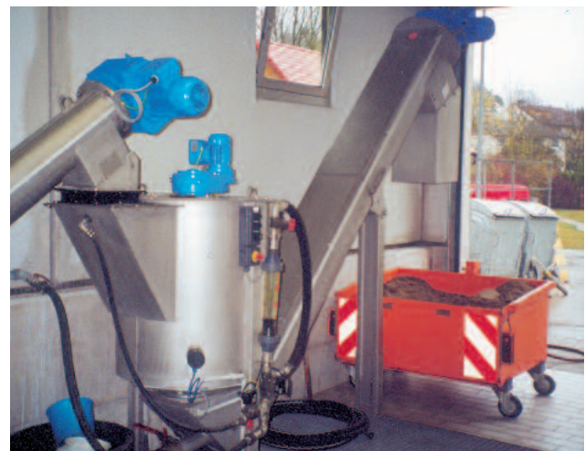
Grit Washer RoSF 4/t fed with classified grit from a ROTAMAT® Complete Plant
