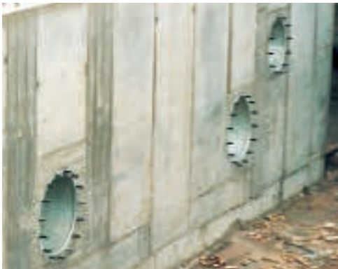
Flush with the wall
