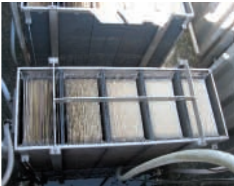
HUBER BioMem® system in container
