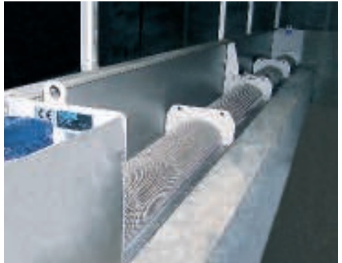
ROTAMAT® Storm Screen RoK 2 installed on foul side of overflow weir
