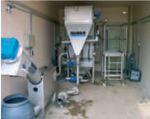
HUBER ROTAMAT® Micro Strainer with 1 mm bar spacing and HUBER Dissolved Air Flotation Plant HDF
