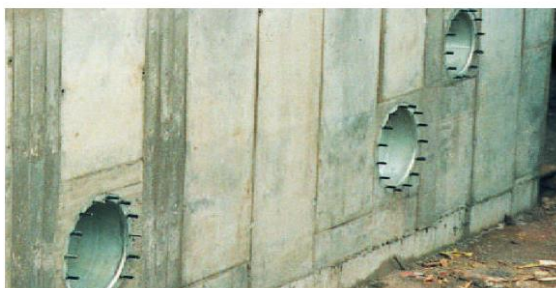
Flush with the wall
