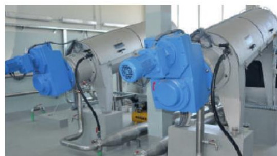
Two HUBER Screw Press Q-PRESS® units installed in parallel
